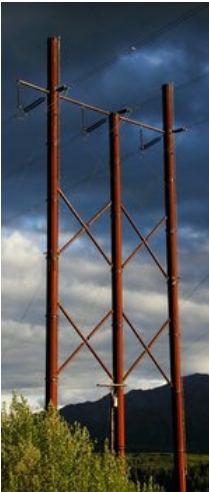
Electrical inertie near Healy, AK
